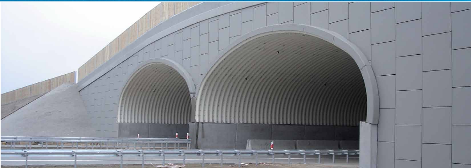
SuperCor® corrugated plate structures and ViaWall A type 1 MSE walls in the WD-10a animal overpass
