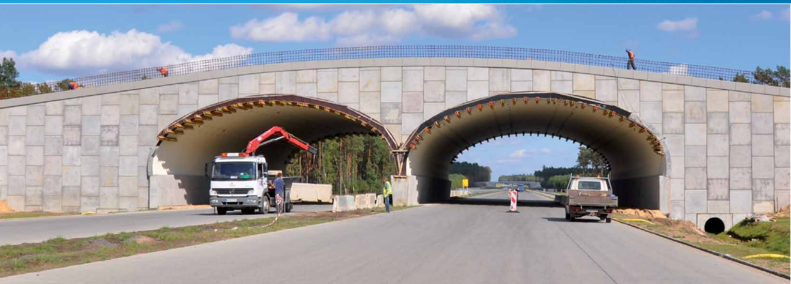
SuperCor® and MultiPlate MP200 corrugated plate structures and ViaWall A type 1 MSE walls in the WD-69a animal overpass
