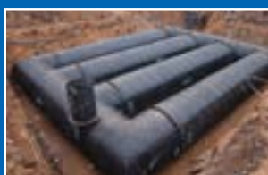
Резервоари ViaWater ViaWater holding tanks
